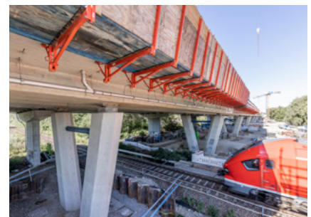
A full enclosure ensures the safety of the traffic below.
